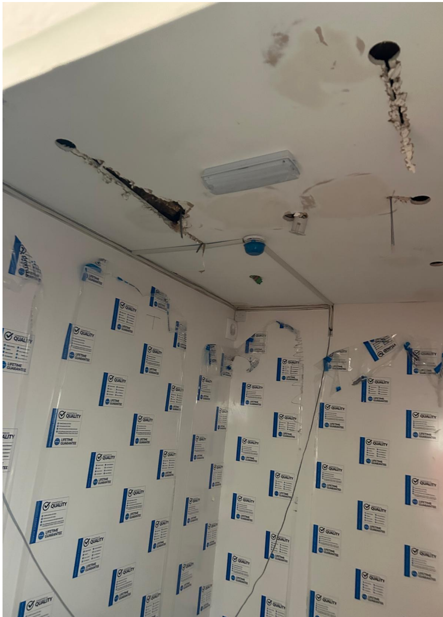
Damaged ceiling and cut wires
