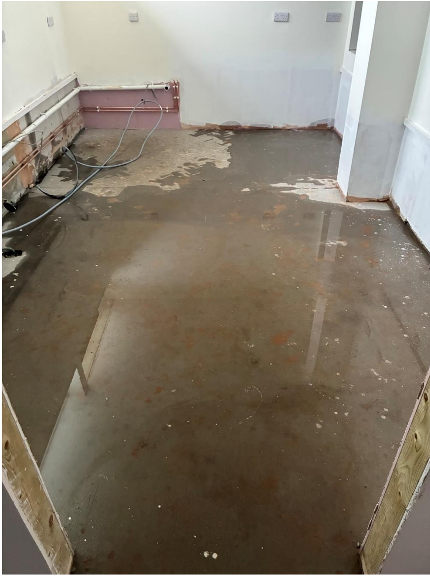
The flooded kitchen floor will need to be replaced
